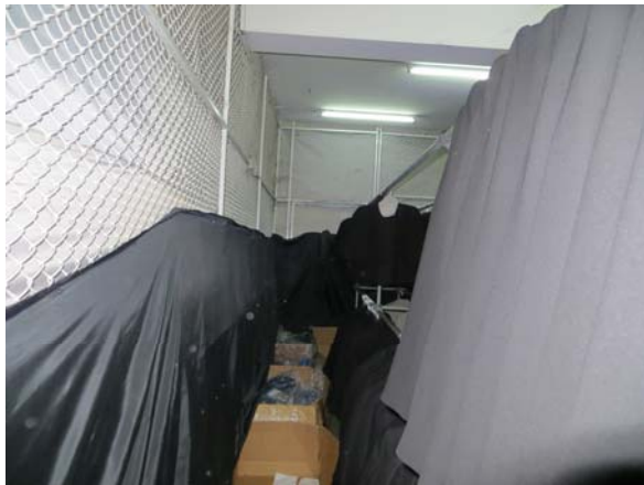
P 12.1 Blocked passageway
