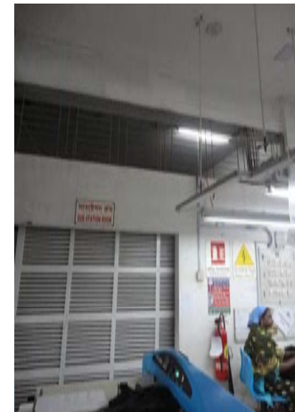
P28.1 Improper separation in substation room
