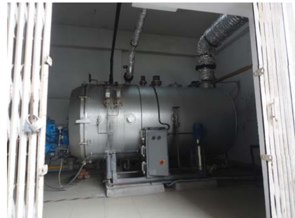
P 23.1 Boiler room is not properly segregated
