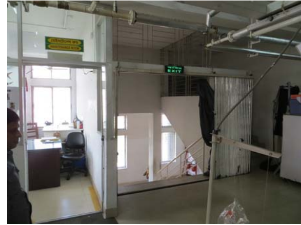
P 11.6 Discontinuous stairway
