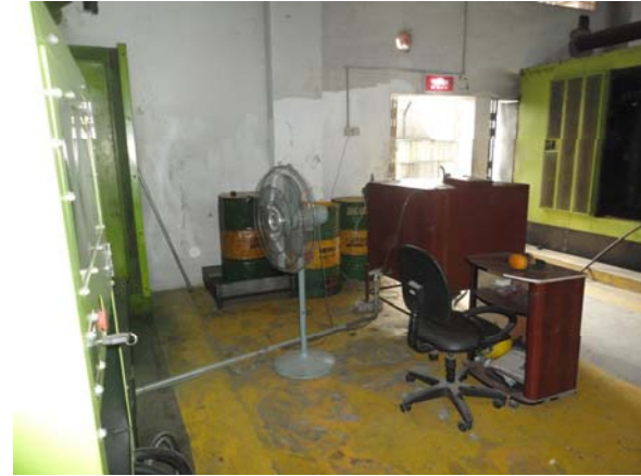
P25.1 Combustible material in generator room
