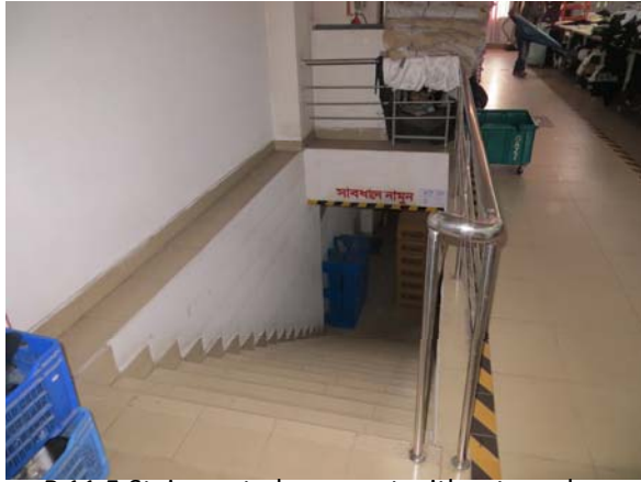
P 11.5 Stairway to basement without smoke-proof enclosure
