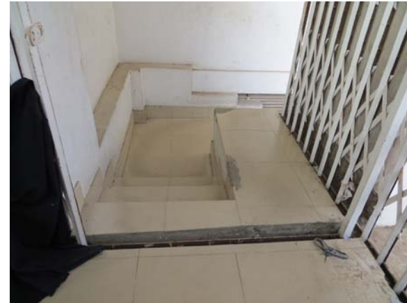
P 11.4 Improperly constructed stairway
