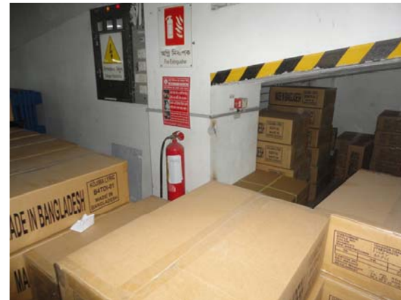
P 19.1 Inaccessible fire extinguisher
