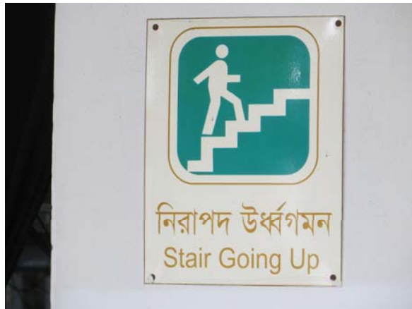
P 16.1 Wrong directional sign
