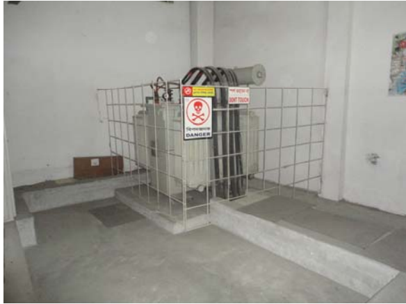
P24.1 No separating wall for transformer
