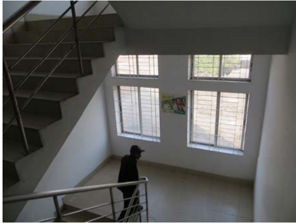
P 11.2 Stairway not in smoke-proof enclosure
